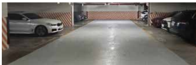
Completed the Epoxy paving project for the B1 parking lot driveway on August 3.
