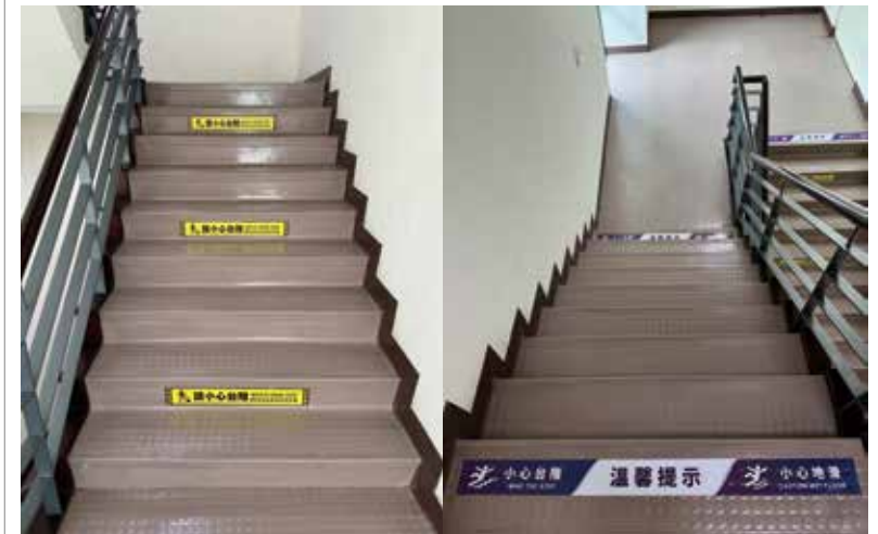
Without safety markings on the floor.
